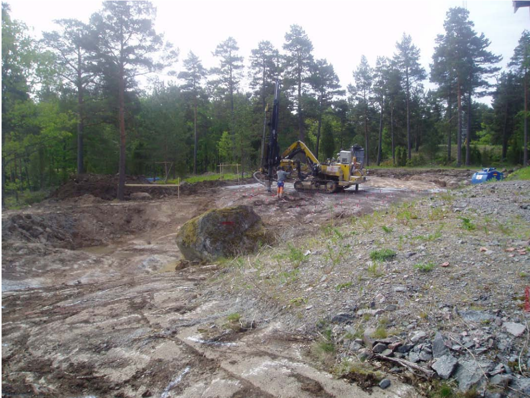
Figure 3-1 The area of the location for the Bentonite Laboratory was uncovered in May and the drilling of holes for the excavation of the rock started in early June.
