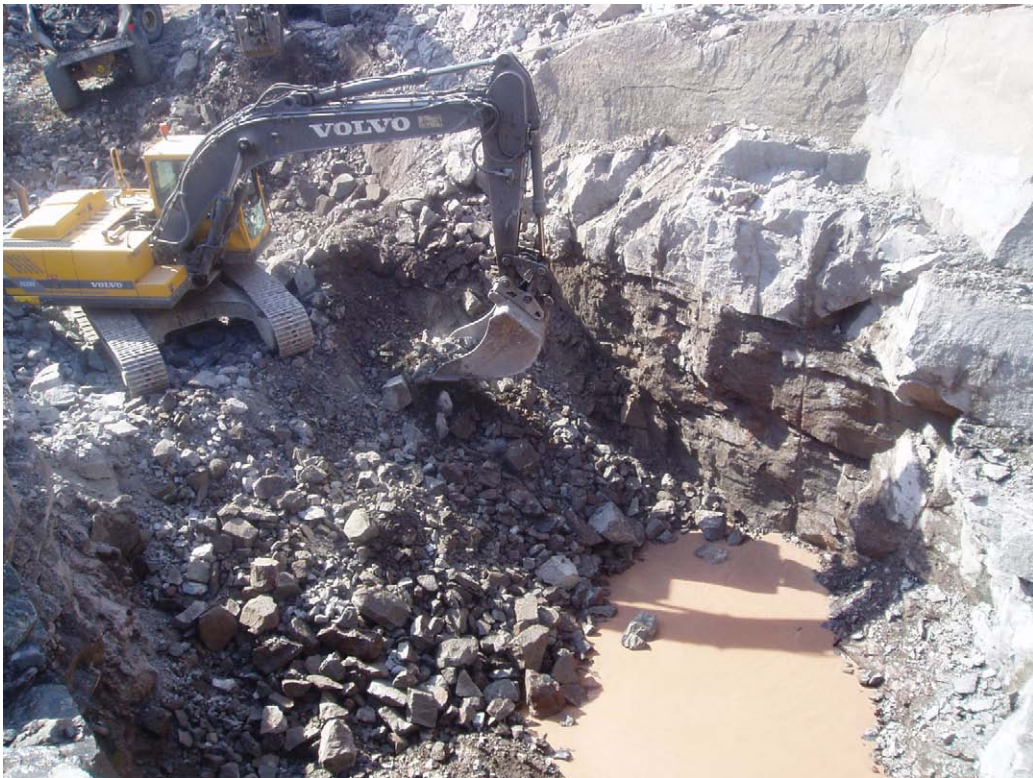
Figure 3-2 The excavated cavity in the rock is about 8 m deep and will host the two deposition holes beneath the foundation slab. The rock excavation work was finalised in the end of June.
